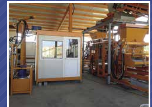
Control cabin with PC and cables of connection of units and assemblies
